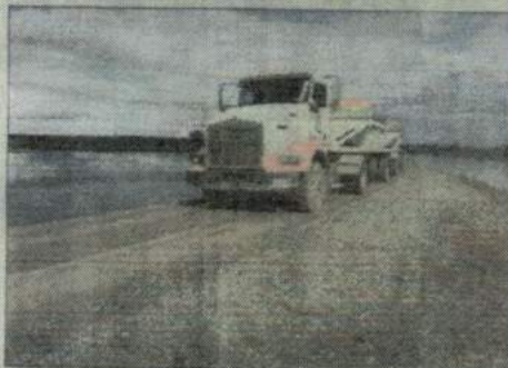
A truck carrying material used to reinforce the site of the breach winds down a narrow levee Tuesday afternoon that has the swollen San Joaquin River on one side and a field that has been inundated.
